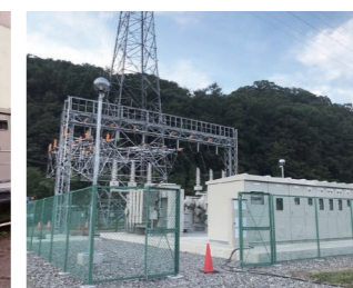
Extra-high voltage substation
