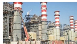
Umm Al Nar Power and Desalination Plant (UAE) ■ On-site construction management ■ Output: 1,550MW (5GT, 2ST Unit)
