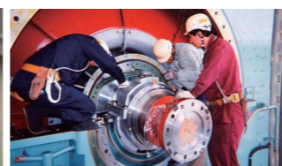
Inspecting a generator
