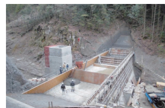
Construction of mega solar power plant and regulating dam H14 m x L51 m x W2 m (dam top), 2,700m 3 of concrete
