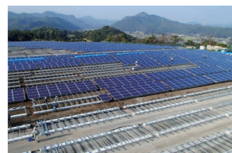
Solar power plant (2,500 kW) (site preparation, foundations, mounting structure, panel installation, drainage, outer fence)
