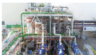
KAWERAU (Geothermal) Power Station (New Zealand) ■ Electrical and instrumentation construction design, material procurement, and on-site construction management ■ Output: 100MW x 1 Unit
