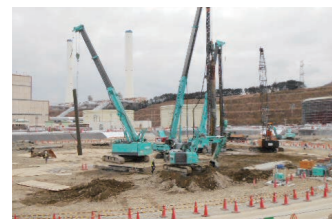
Removal of oil tank foundations and other items Breaking foundations and removing piles
